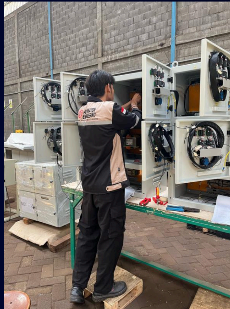
Wiring Panel MCC
