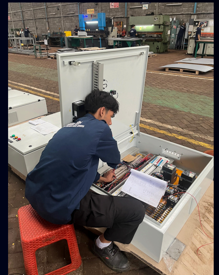
Quality Control Panel DB
